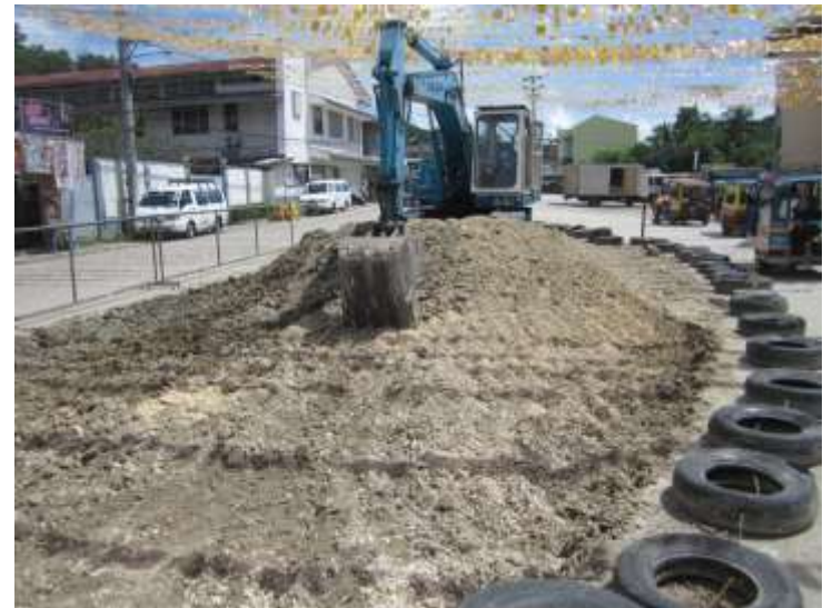
Concreting and cementing of the kiosk side of the Jagna Business Center
