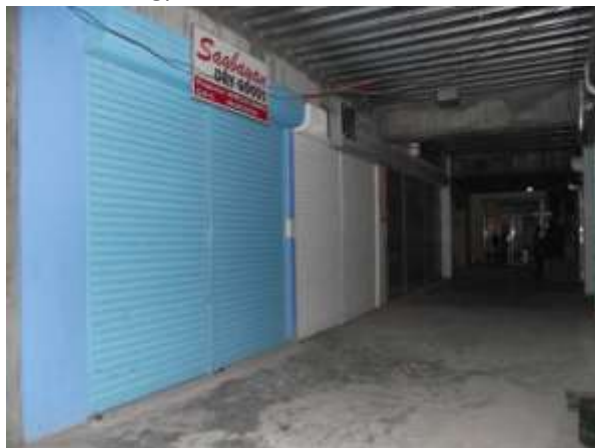
Stall division and roll up door provision at the Jagna Business Center
